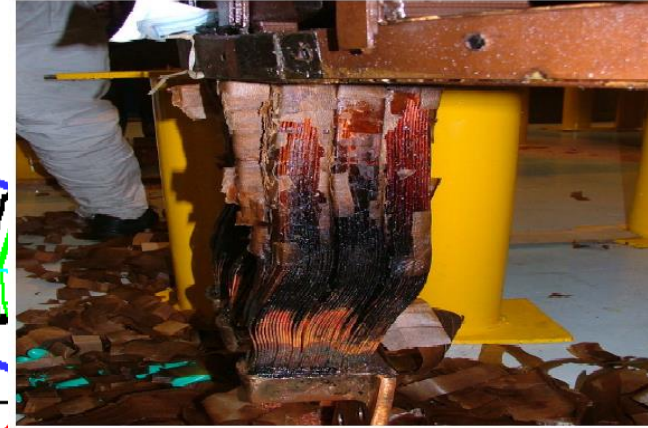
Station 3 Transformer 6 LV exit lead overheating
