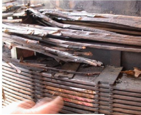
Station 4 Transformer 6 HV winding failure
